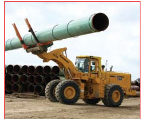
Extreme care has to be taken with handling the coated pipe. Damage can occur simply by the way the forks grab them.
