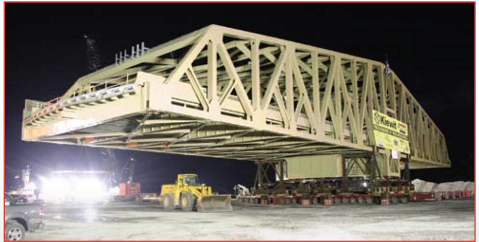
The swing span for the Willis Avenue bridge in New York City was constructed by Kiewit and D.A.Collins at the Port.
